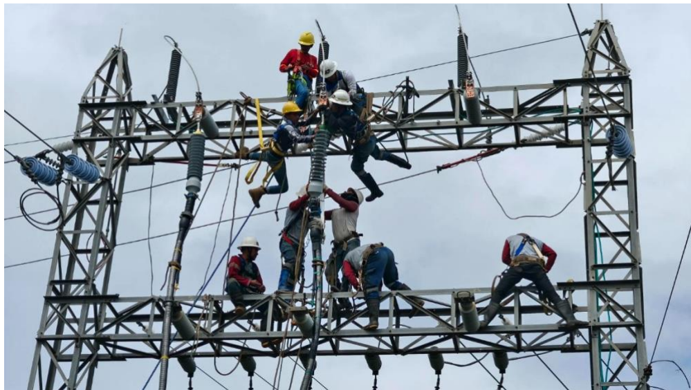
NGCP completed the rehabilitation, repair, and reconductoring of the Unidos-Caticlan 69kV Line ahead of the March 2026 target.
