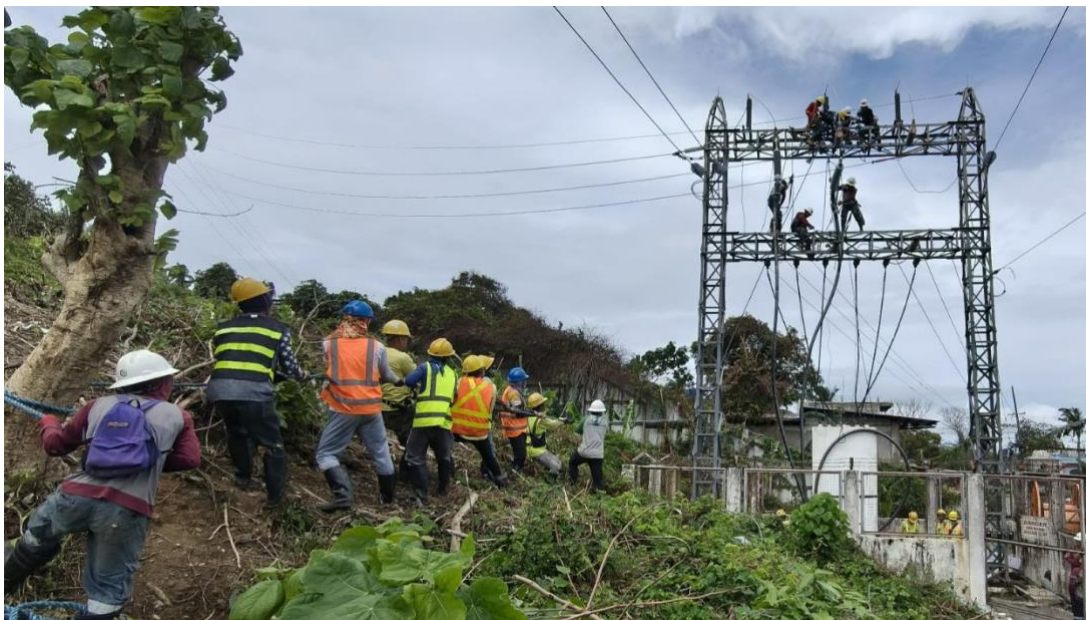
NGCP deployed augmentation teams from South Luzon and other parts of Visayas to fast track the replacement of the Unidos-Caticlan 69kV Line.
