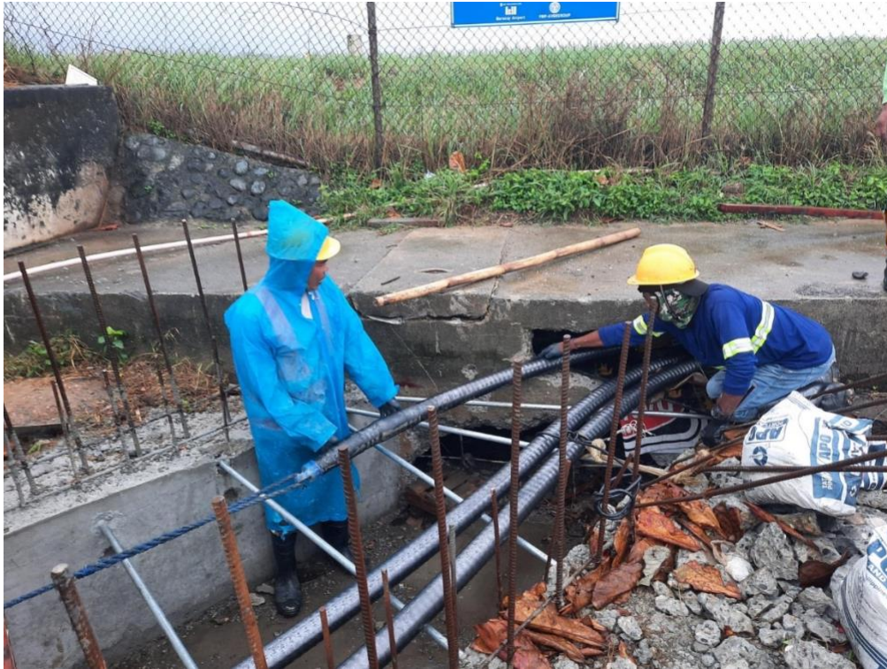
Despite inclement weather and technical limitations, NGCP line personnel continue replacement works on the 69kV underground cable.
